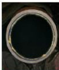
Liner tight fit
