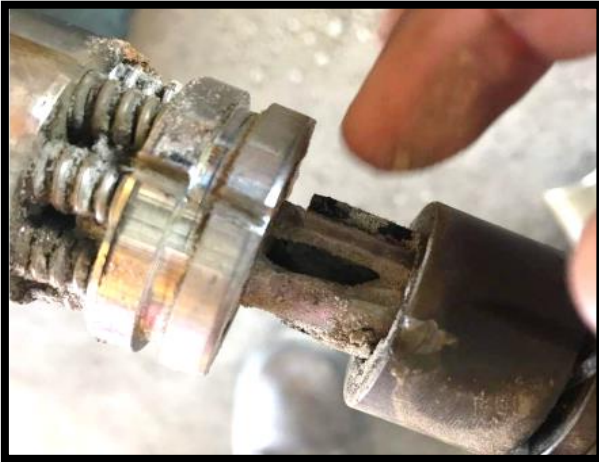
Base pipe erosion at spring compensator area
